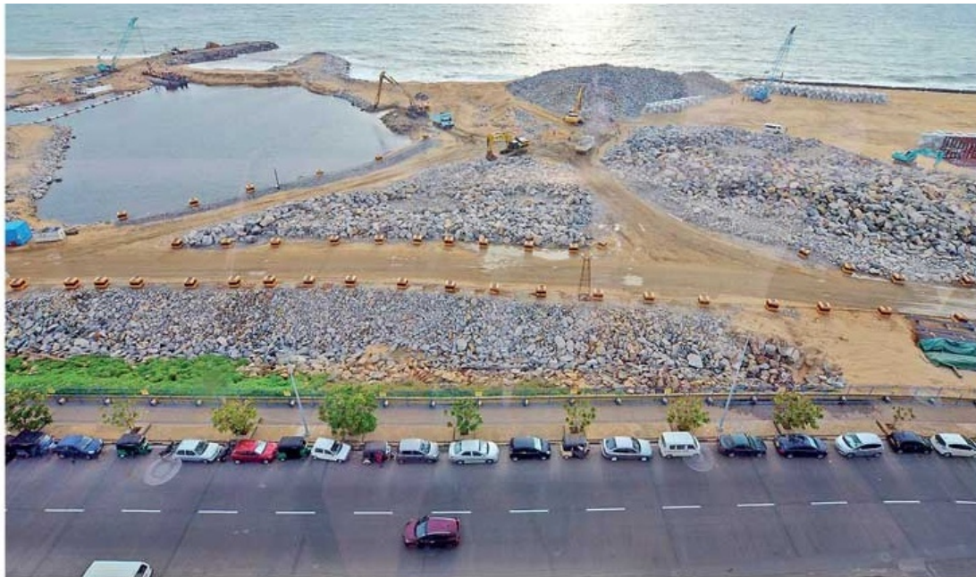
Over 40% of Colombo Port City is now reclaimed – Pic by Shehan Gunasekara
